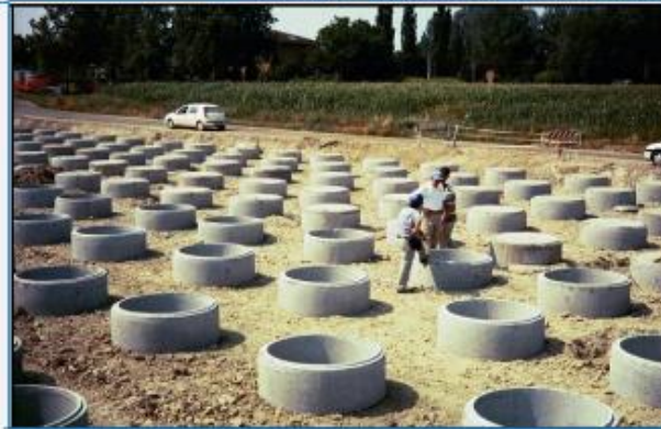
CFA to support an Embankment Square RC Precast Driven Piles to support an embankment
